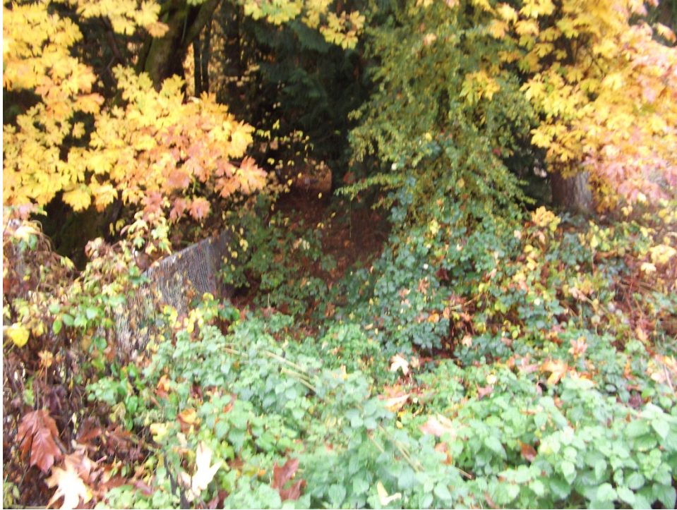
The natural drainage channel on the south side of NE 100 th St. ❶
